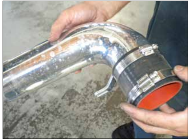
o. Install a straight coupler and two hose clamps onto the lower pipe.
