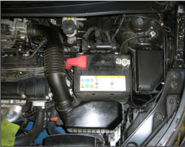
Factory airbox system installed
