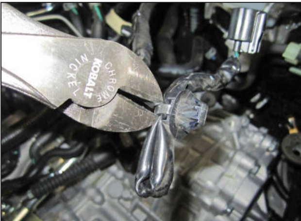
u. Cut and remove the clip from the MAF sensor harness as shown. NOTE: Use caution and DO NOT cut the MAF sensor wire harness.
